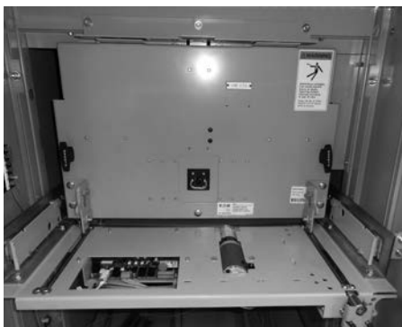
Type VCP-W Standard Switchgear Auxiliary Drawer with Type MR2 Integral Racking
